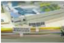
Fibre optic cable markers
