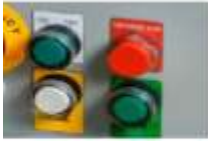
Control panel labels
